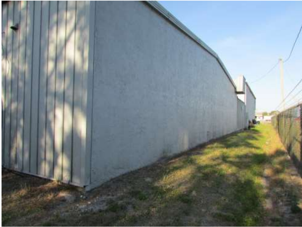
Rear view of the administrative building and the apparatus bays (Photo Taken on April 6, 2021)
